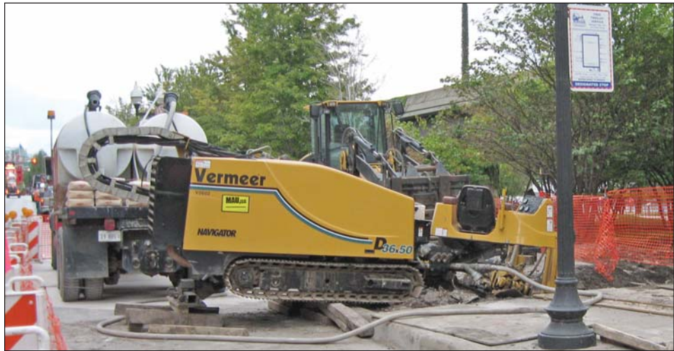
Due to extremely tight space restriction, Mid America was forced to use a smaller HDD rig. However, the two bores were still accomplished on schedule.
