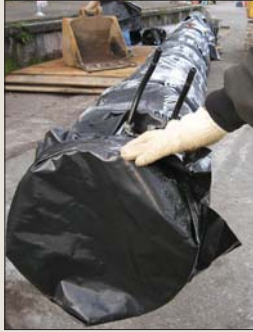
Fig 5 (left): Bonding wires installed across each pipe joint creates a continuous electric circuit between corrosion test stations. Photo courtesy Portland Water Bureau. Fig 6 (right): Polyethylene encasement provides additional protection from corrosion. Photo courtesy Portland Water Bureau.
