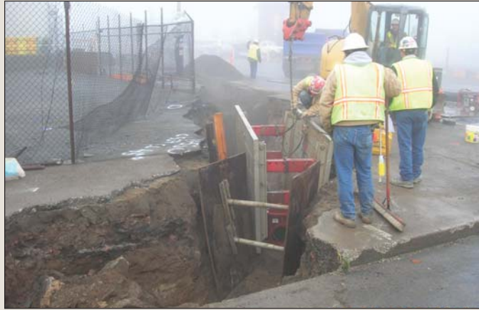
Fig 1: Shoring can prove to be challenging in streets that are congested with other utilities. Photo courtesy of Portland Water Bureau.
