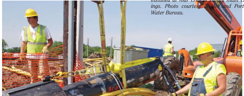
Fig 3: Concrete-encased HDPE pipe provides a cost-effective alternative to steel-encased pipe. Photo courtesy TriMet and Portland Water Bureau.
