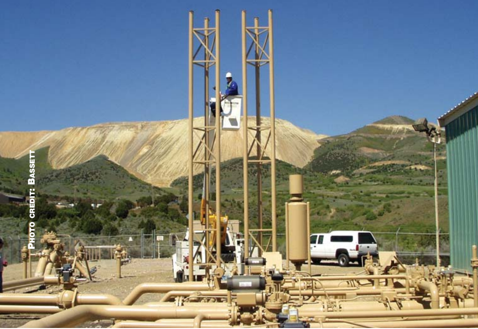
Men and equipment working at Questar Pipeline's interconnect with Northwest Pipeline in northeastern Utah.
