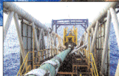
A 20-inch joint of the export line is visible in the stinger of the derrick lay barge.
